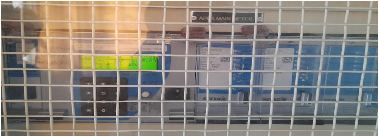
Main meter and check meter.
